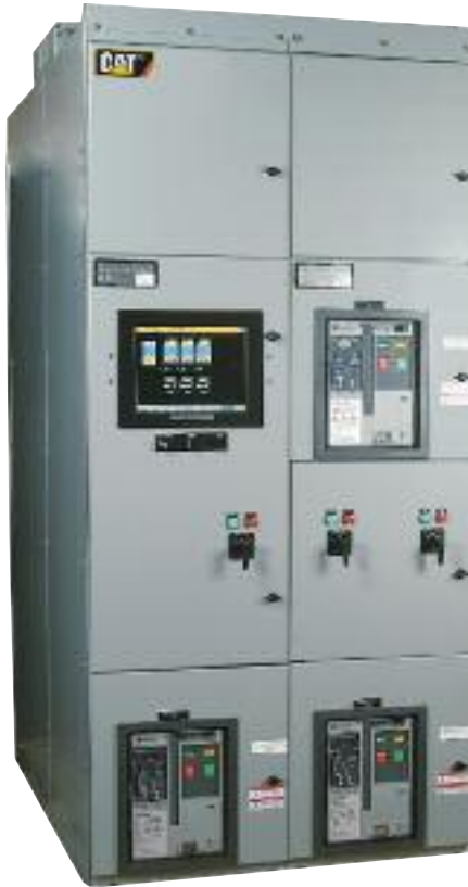
This switchgear from Caterpillar Inc. can be configured for emergency generator paralleling or emergency transfer and load management.
